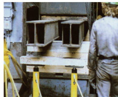
Replacing adjustment rolls under a fly-over with RR cylinders, for controlled lifting an lowering.
